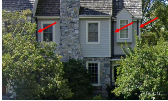
Berks County home where indicated downspouts were creating mosquito habitat
